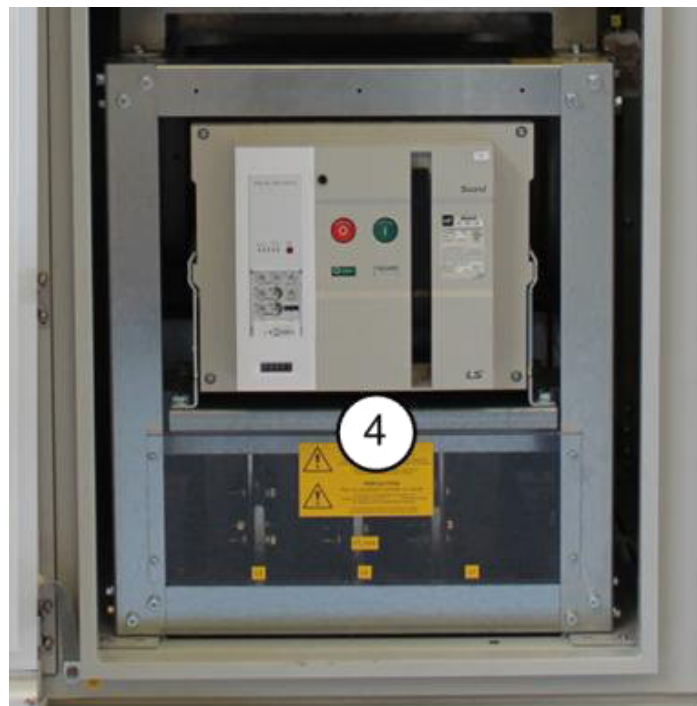
Figure 3.4 Main AC circuit breaker
