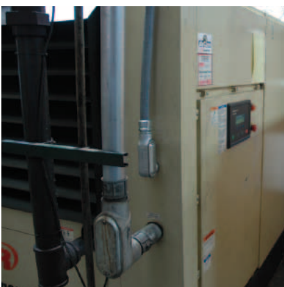
Air Compressor Control
