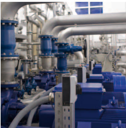
Industrial Pump Control
